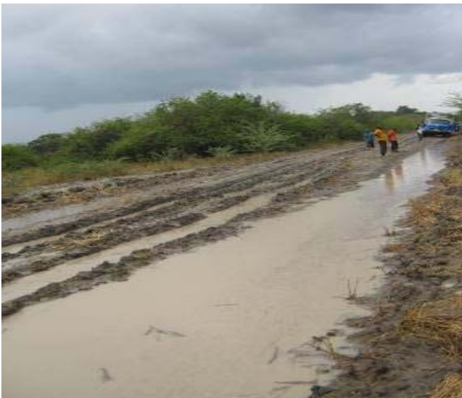
Completely stuck on the muddy water-logged road!
